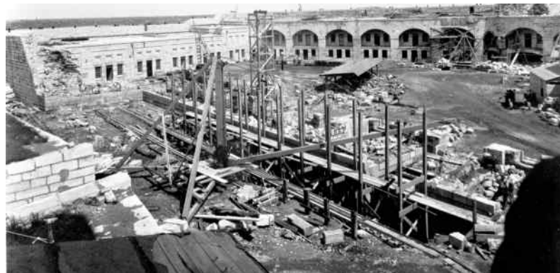
Figure 8. The reconstruction of the curtain wall during the 1936-1938 restoration. Fort Henry Archives.
